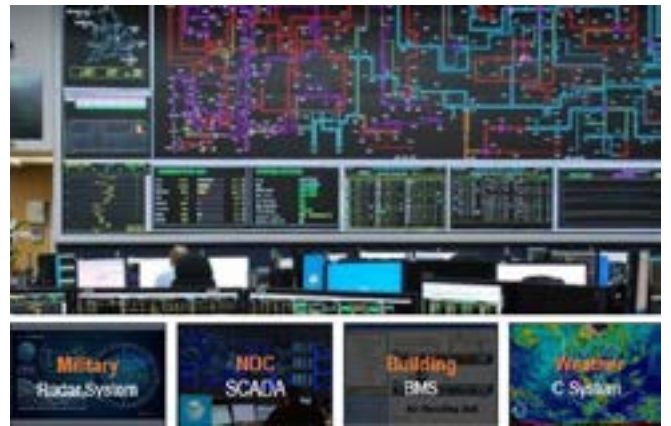
Figure 4 SCADA system screen for utilities and power plants
